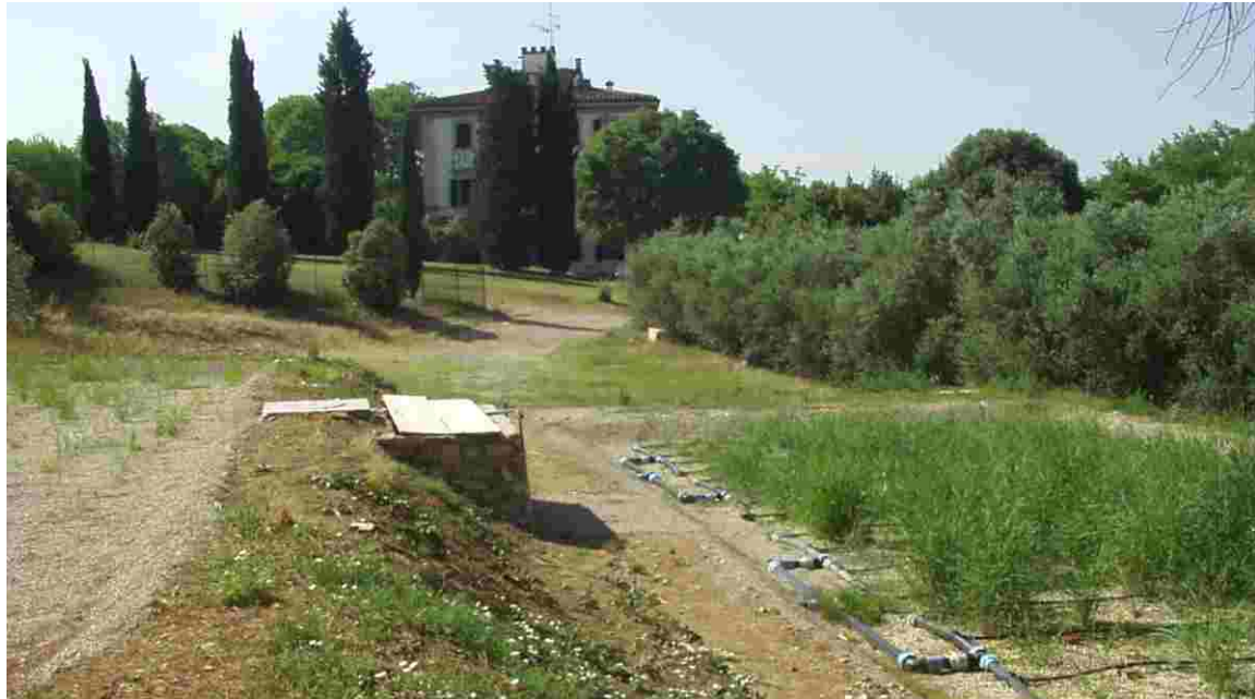
Detail of a multi-stage system consisting of a horizontal subsurface flow system (right) and a vertical one (left) at the service of a tourist structure - 140 equivalent inhabitants (Florence, Italy)
